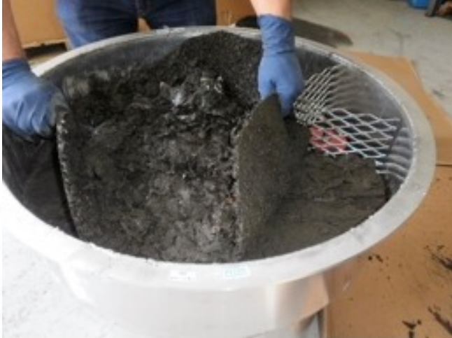
The first filter layer, a plastic mesh called flow free, is removed. The filter is totally clogged with mud, grease and dirt.
